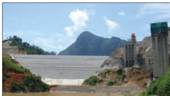
The 50 MW Nam Lik 1-2 scheme in Laos. The first two schemes which were financed entirely for domestic supply within Lao PDR.
