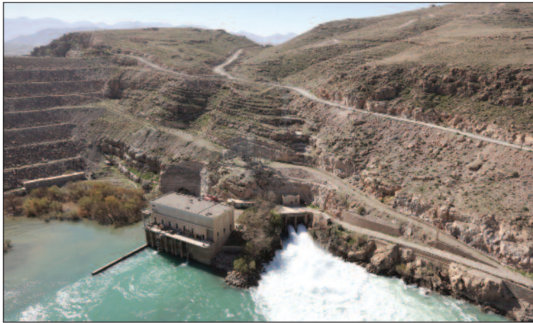
The Kajaki dam and powerplant, which supplies electricity to Kandahar. A major military exercise was required to bring a runner to the site for refurbishment in 2008.
