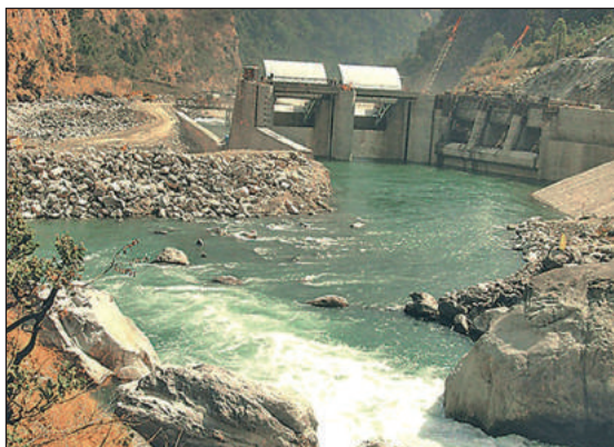
Site of the Upper Trishuli project, for which a PDA was recently signed (see details on p20).
